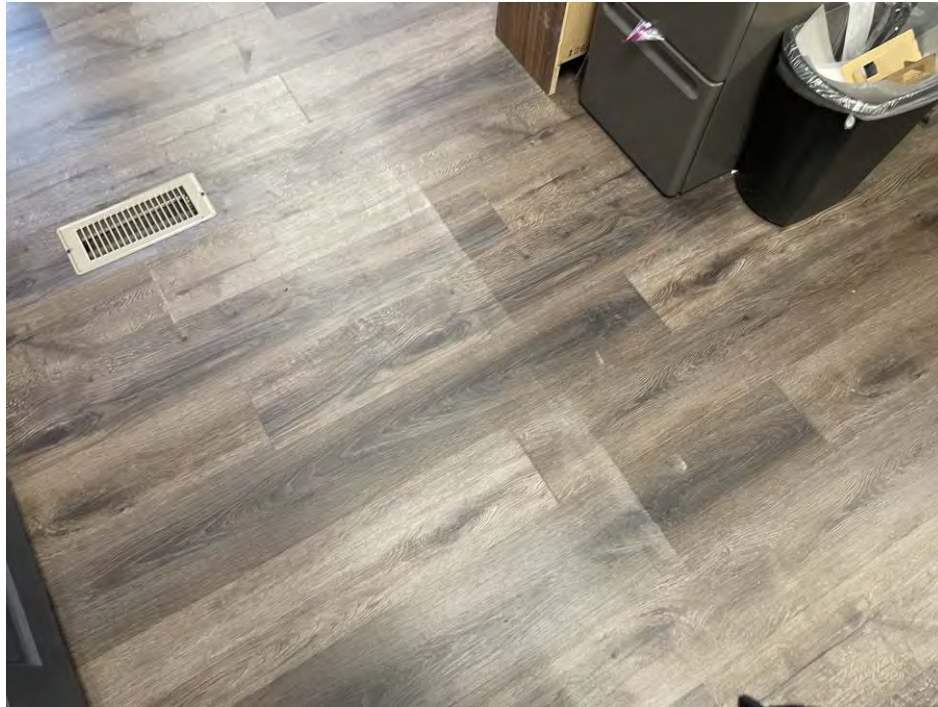
Photo 3. Line laminate flooring indicates some sort of movement in floor framing. See photo 4.
