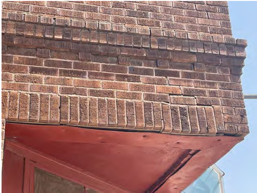
Photo 11. Front entrance area. Gaps between steel plate and the bottom of brick have cause the brick to settle in some places. Fill area between steel plate and bottom of brick with mortar and continue to monitor the plate for additional movement.
