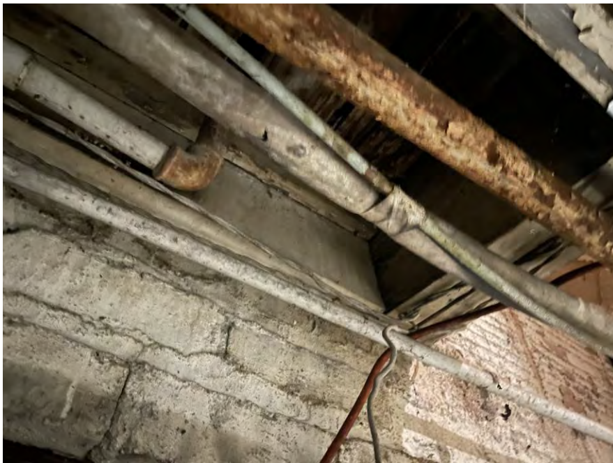
Photo 6. Basement stair framing opening on south side. Wood framing stops at wall and does not bear on wall. Framing is unsupported and is loadbearing.
