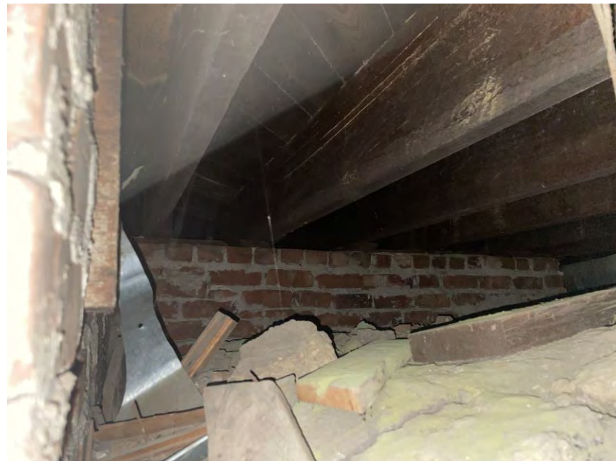
Photo 4. Crawlspace looking northeast. Gaps noted between bottom of floor joist top of brick wall which likely creates lines under laminate.
