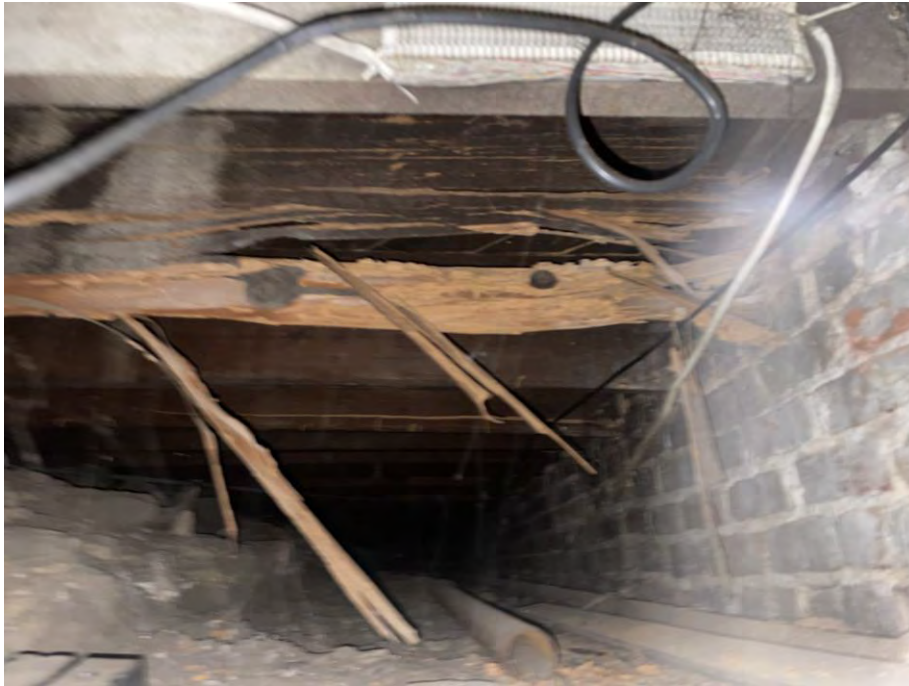
Photo 5. Crawlspace view from south wall. Joist is shredded at the wall interface. Replace or sister floor joist and attach to brick wall.
