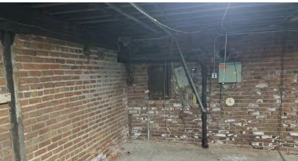
figure M1 - sanitary and vent piping in basement
