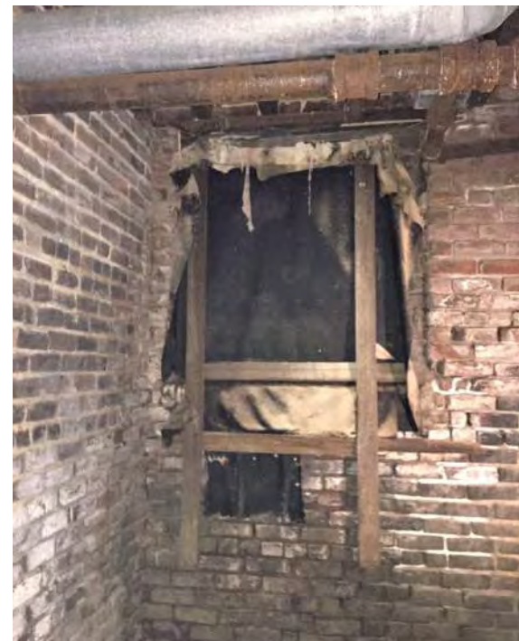
figure A07 - abandoned opening in mechanical room
