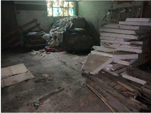
7 Debris pile in vacant south building.
