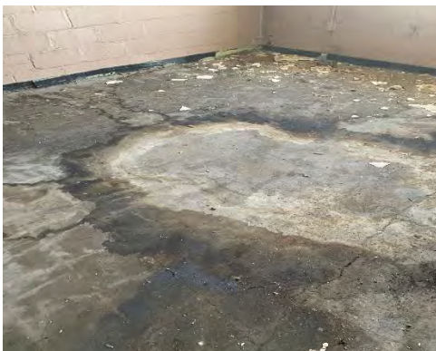
5 Staining on floor in vacant south building.
