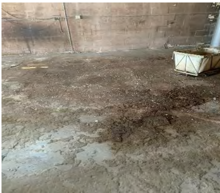
3 Unknown debris on floor in vacant south building.
