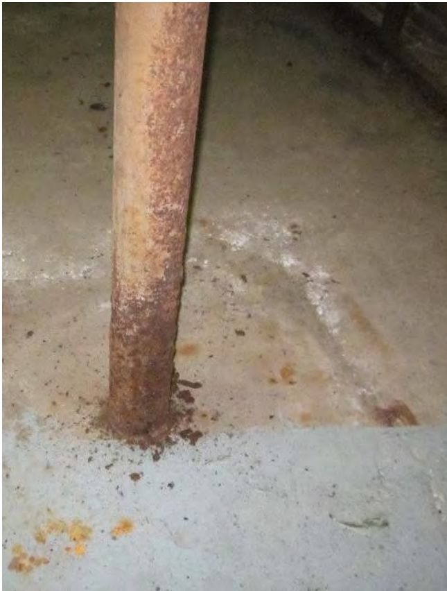
figure S6 - rust at steel column
