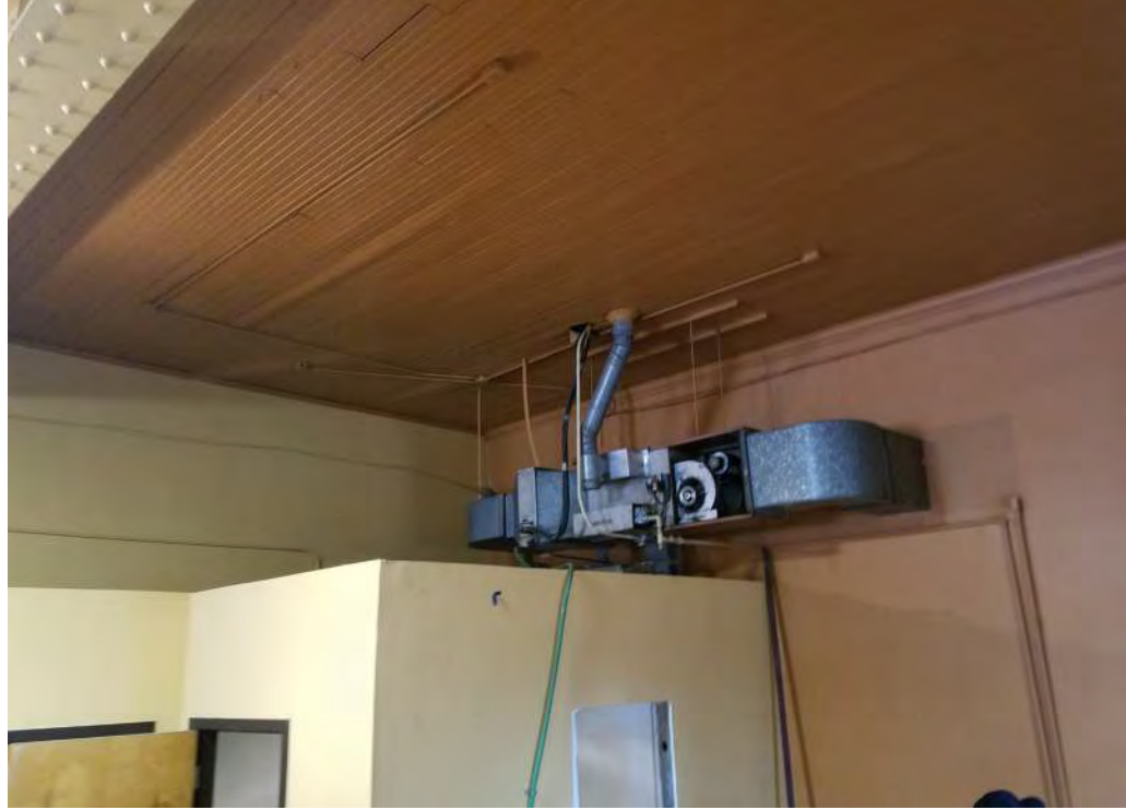
figure M6 - HVAC system serving North portion of building
