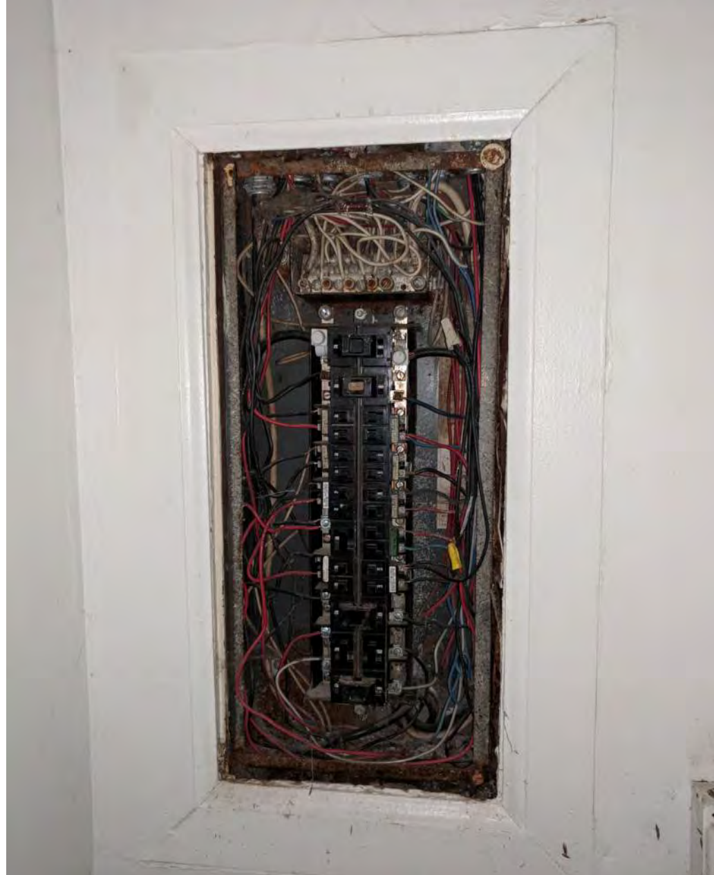
figure E2 - main electrical panel
