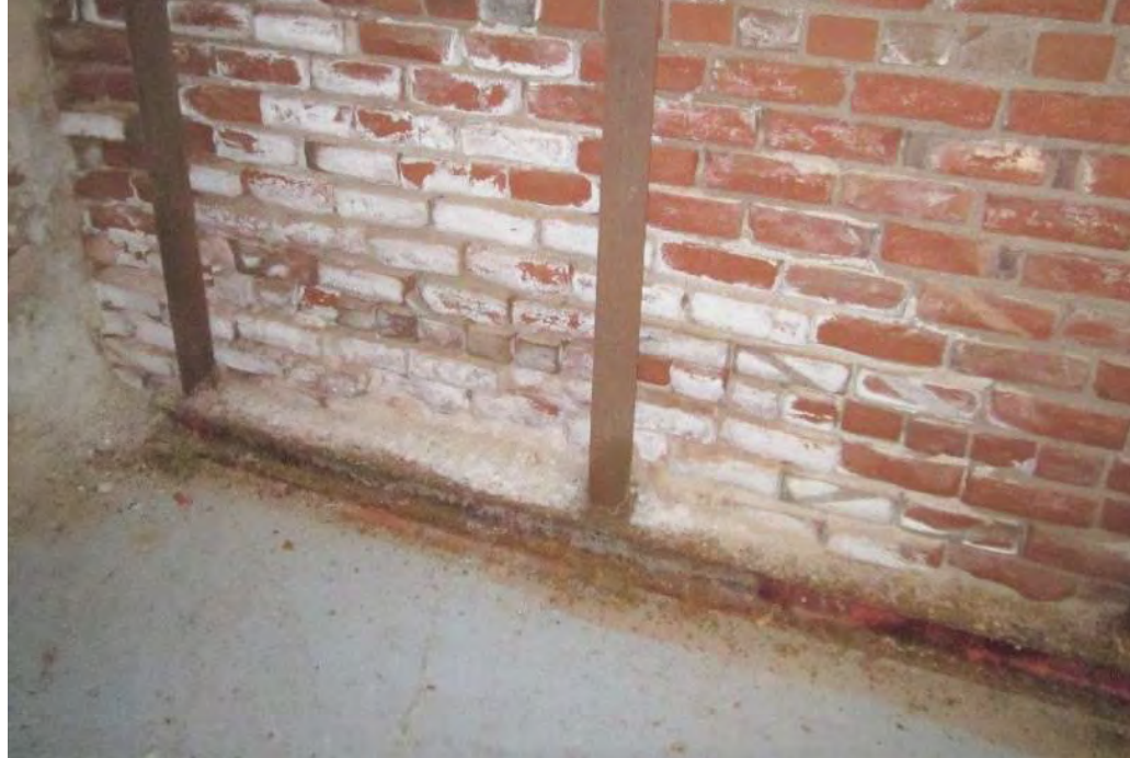
figure S5 - efflorescence resulting from water infiltration
