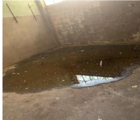
2 Pool of liquid in vacant south building.
