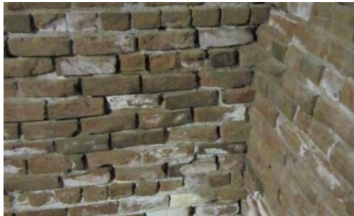
figure S4 - interior masonry in need of repointing
