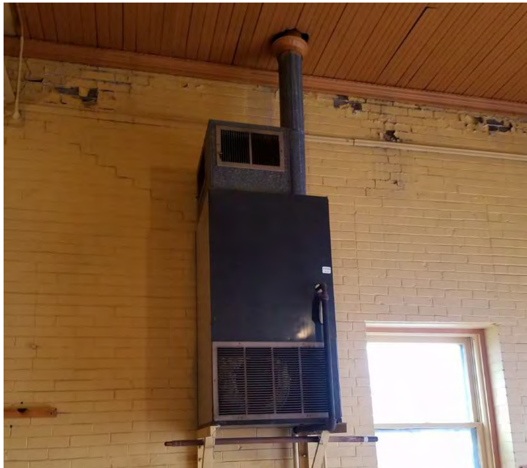
figure M7 - heating system serving garage area
