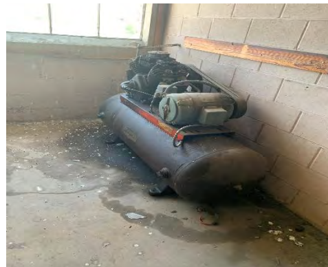
4 Air compressor in vacant south building.
