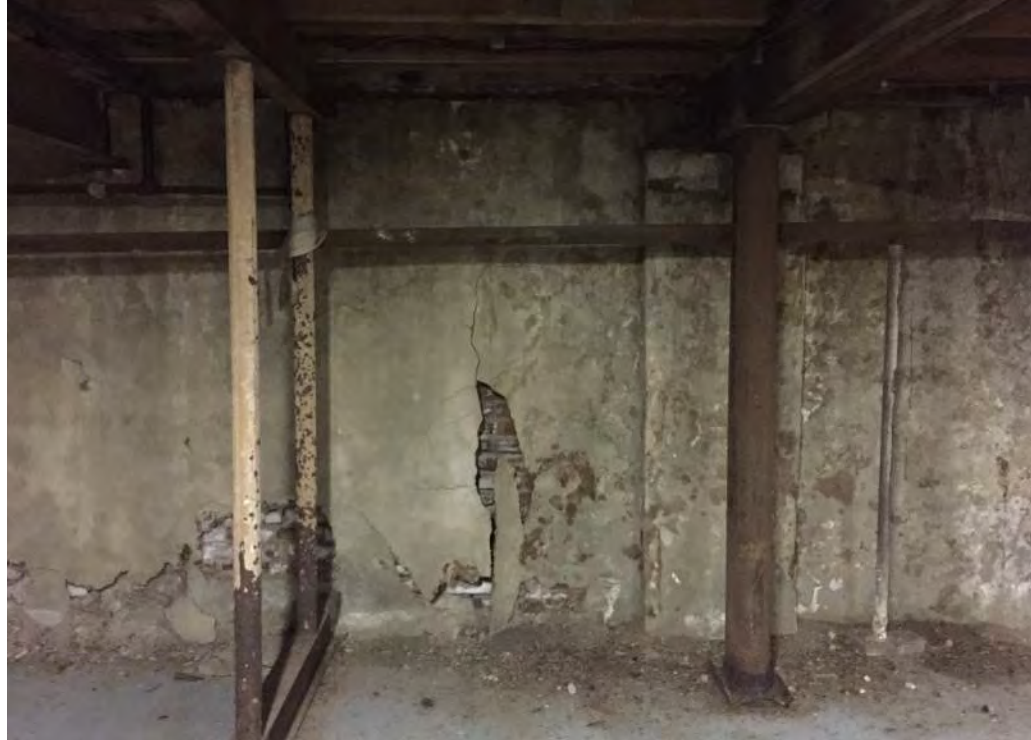
figure A06 - plaster at south basement exterior wall
