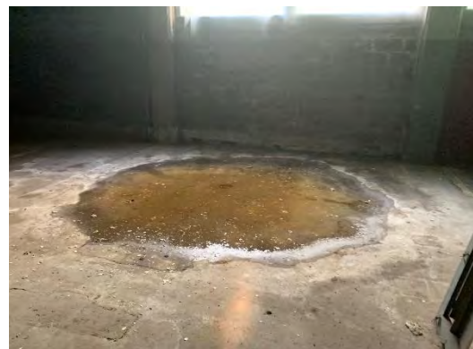
6 Pool of liquid in vacant south building.
