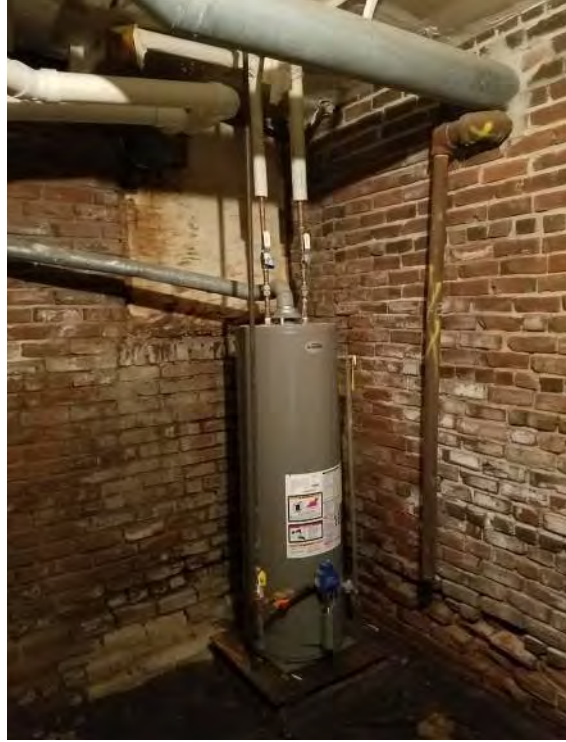
figure M4 - existing water heater
