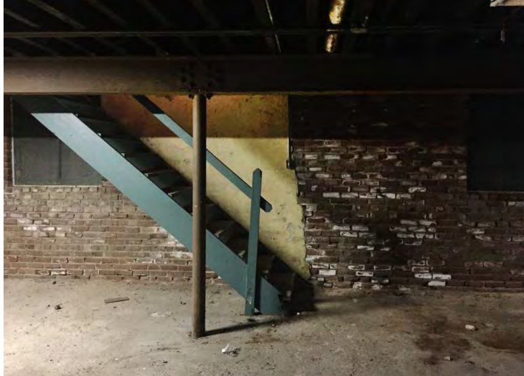
figure A10 - wood stair, iron column and beam, abandoned windows
