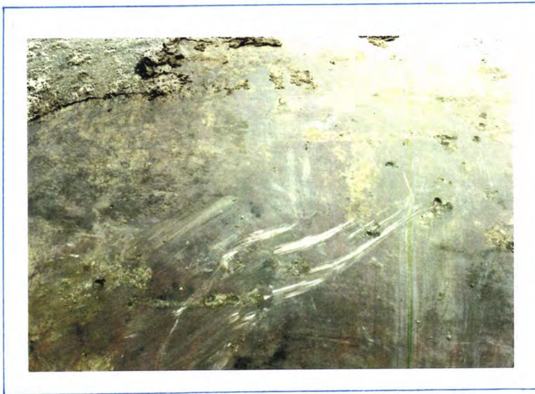
Photo #2. Corrosion pits are found in many places on the west end of the tank. None of these pits were found to penetrate the tank shell.
