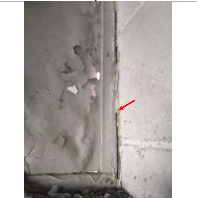
Sample #8 (interior window frame caulking). Tested positive for asbestos.
