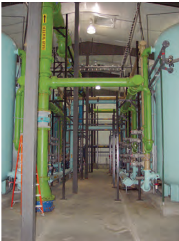
Ion Exchange plant to remove nitrates (McCook, NE).
