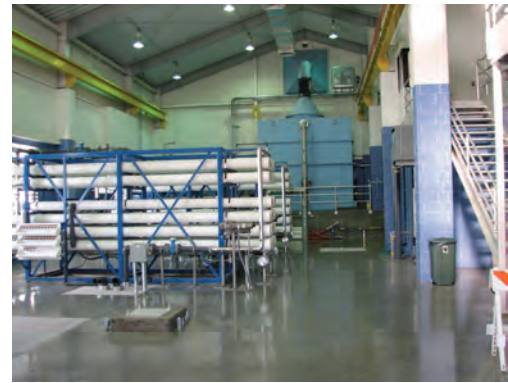
Reverse Osmosis treatment plant to remove nitrates (Seward, NE).
